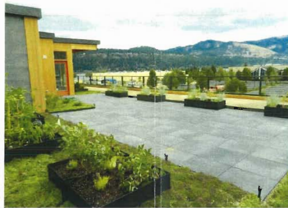
ROOFTOP COURTYARD PAVERS AND SEDUM CARPET
